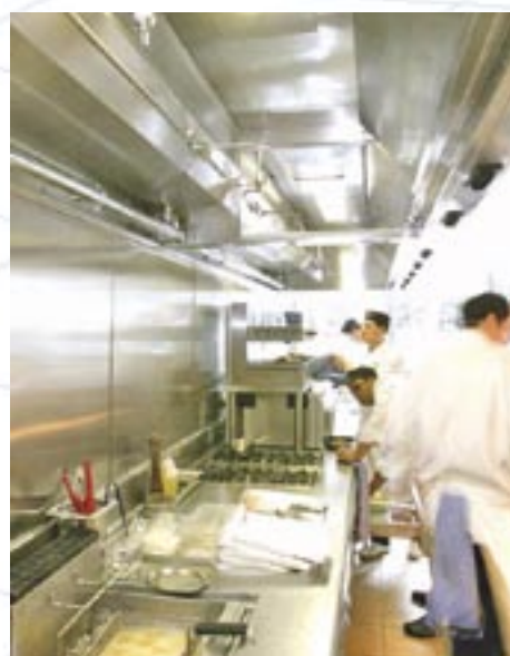
Water Wash Canopies, Marriott International, U.K.
