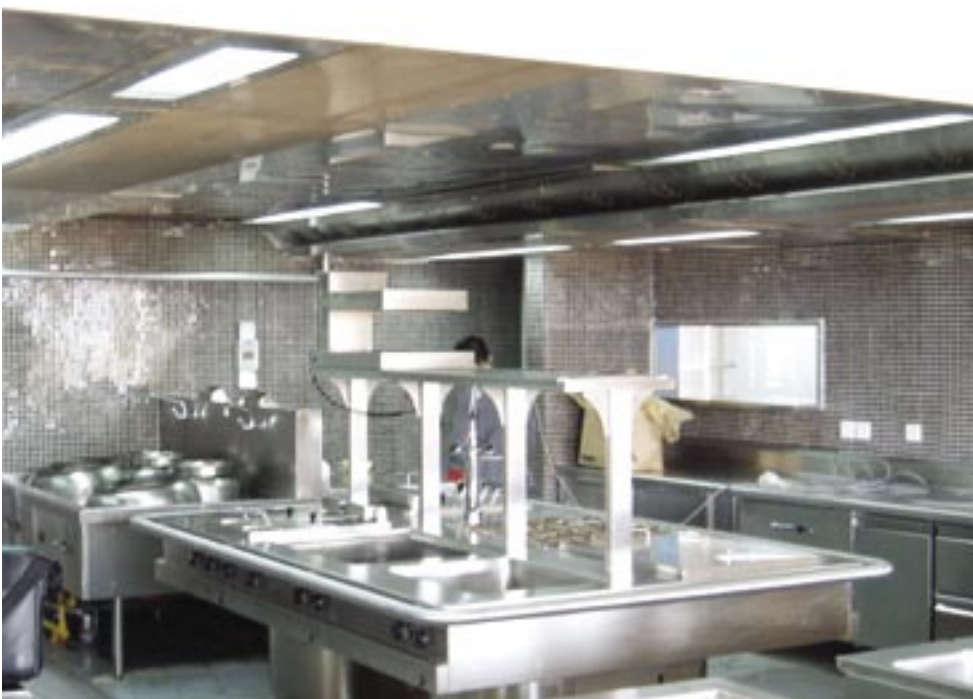
Water Wash Ceiling, Puzhou, China
